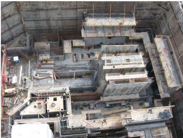
intelliRock sensors are placed in the center and face of each wall pour to monitor the temperature differential.
