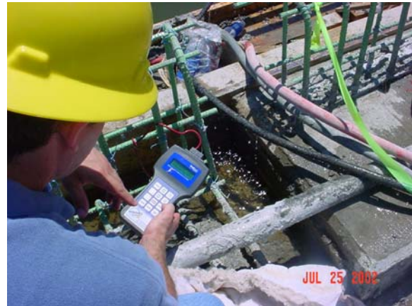
An engineer takes a strength reading at the I-40 bridge construction site using IntelliRock.
