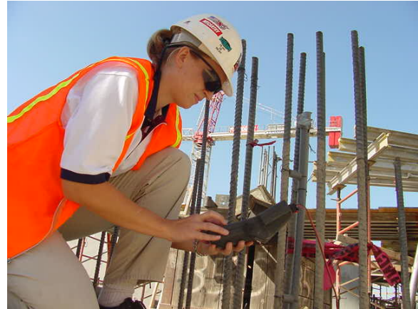
McCarthy Project Engineer Pamela Culbertson uses intelliRock to take a strength reading at the 4 th Avenue Jail project site.
